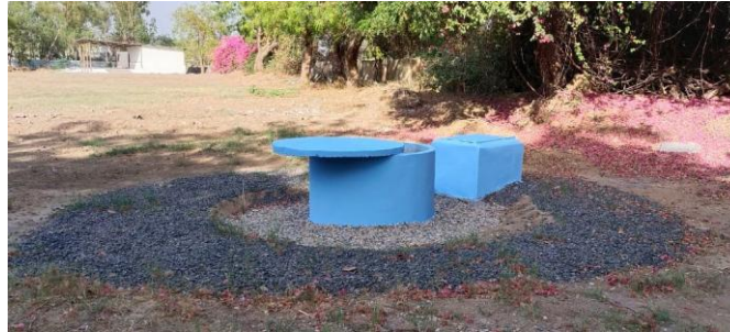
Scientifically Designed Recharge Well System
